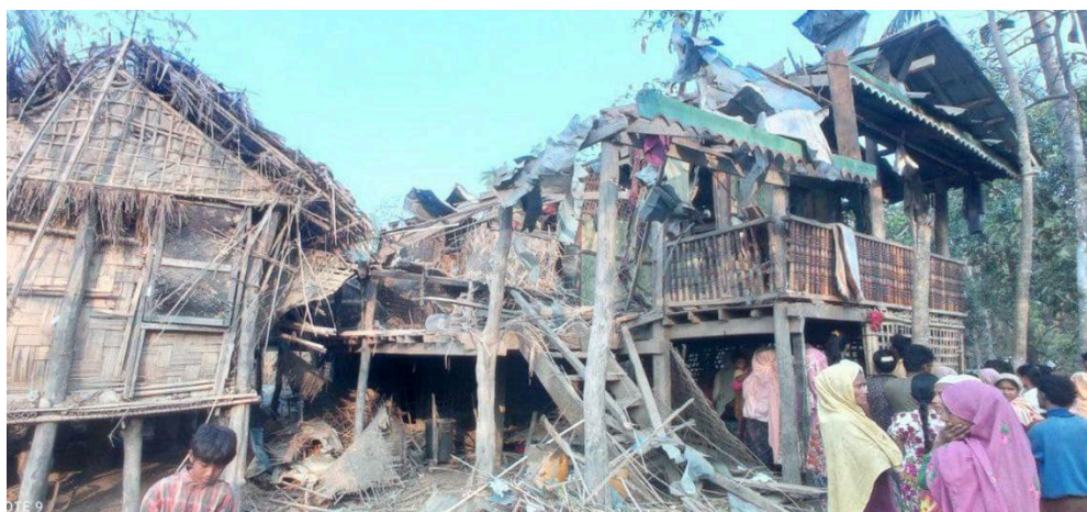
A house destroyed by the Burmese military's airstrikes on Thar Dar village, Minbya township, Rakhine State, on March 18, 2024. 96
