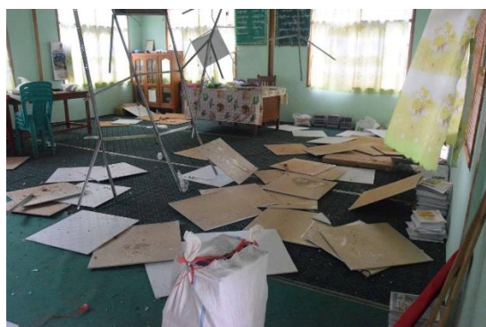
School damaged by SAC airstrikes
