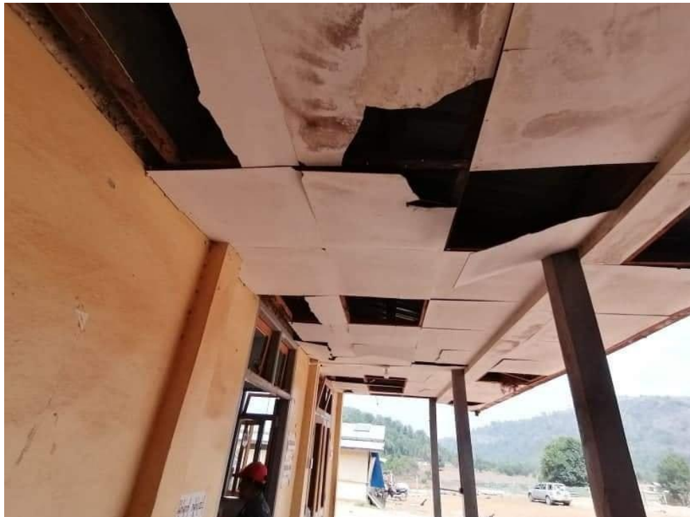
Figure 4: Images showing roof damage at the same site. (Source: Khit Thit Media ).
