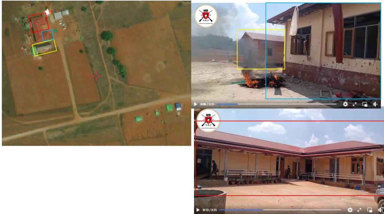
Figure 3: Images showing damage to the structure. (Source: Moby People Defense Force ).
