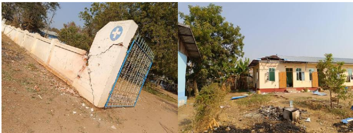
Figure 2: Imagery allegedly taken after the airstrike on Ma Le Thar. (Left) Damage to the hospital wall (22.113461, 95.452112). (Right) Damage to a nearby medical facility building (22.114029, 95.451988) (Source: Ayadaw Post ).
